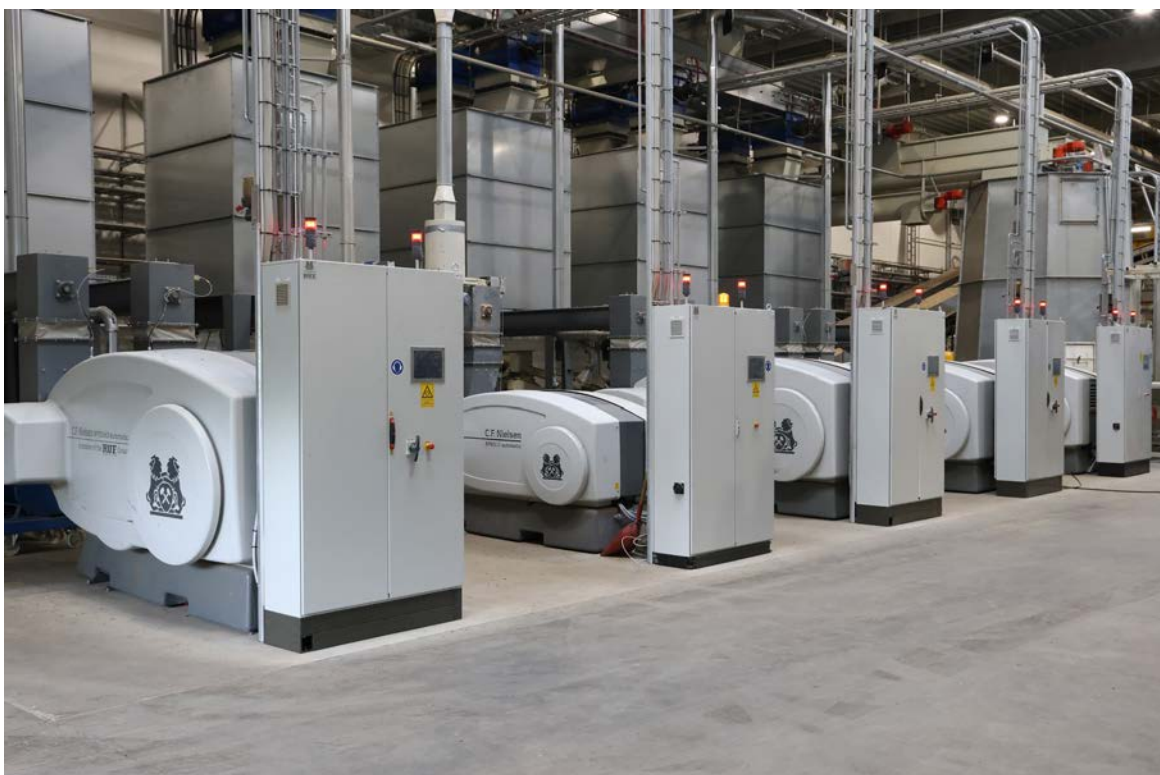
A 5 presses installation at a larger producer of briquetted straw for bedding and biogas plants.
